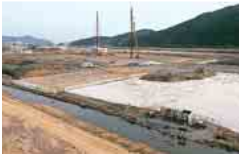
Menard Vacuum Treatment™ to preload 40 m of very soft marine mud at Pusan (South Korea) sewage treatment plant. View of the membrane during the Vacuum application.
