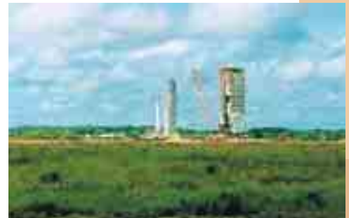
Installation of Dynamic Replacement Pillars under the Kourou Railway (French Guyana) between Ariane 5 construction area and launching pad.
