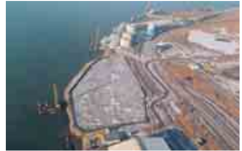
Port of Wismar (Germany) - Pre-consolidation of the TPC (22,000 m 2 ) using Menard Vacuum Consolidation™.
