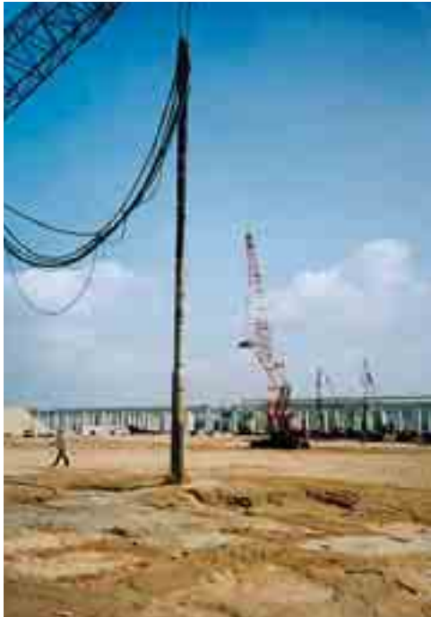
Treatment to a depth of 15 m using vibro compaction in Pasir Pajang (Singapore).
