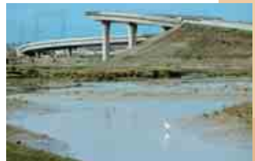
Soil Improvement by CMC™, below access embankments to bridge. View of site after erection of fill.
