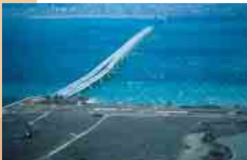
Consolidation by Dynamic consolidation in Osaka (Japan) airport's artificial island using a Tripode with 1400 TM energy (drop height times pounder weight).
