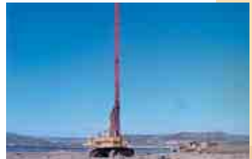
Installation of vertical drains at 25 m depth in clay under the Rabat-Larache expressway (Morocco) to consolidate the road embankments by preloading.
